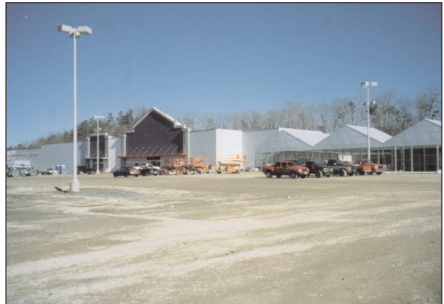
Lowe's store under construction in East Ellijay shown here in late January.
